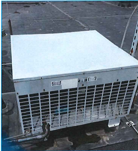
Existing condensing unit
