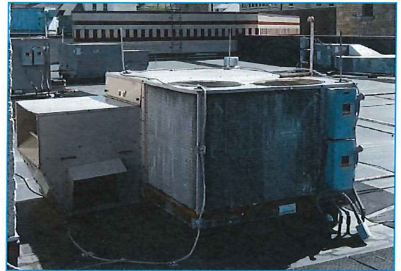
Typical Packaged Rooftop Unit
