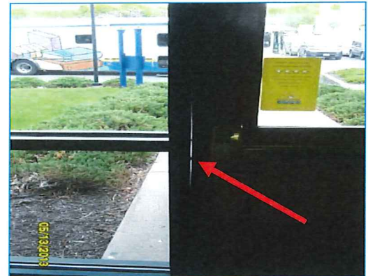
Gap from deteriorated door seal at Visitors Center
