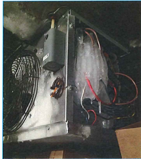
Existing evaporator with frozen coil in freezer. The ice prevented the fan from operating properly
