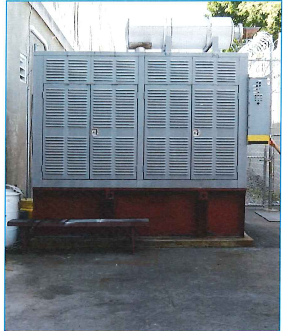
Existing 400 kW emergency generator
