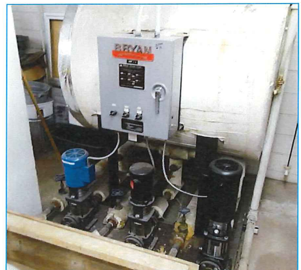
Steam Condensate Receiver & Pumps
