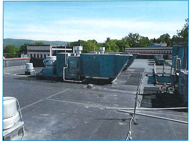
Existing hood make up air units
