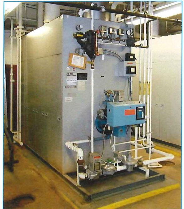
Existing Bryan Boiler
