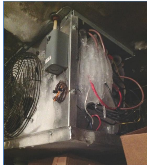
Existing evaporator with frozen coil in freezer. The ice prevented the fan from operating properly
