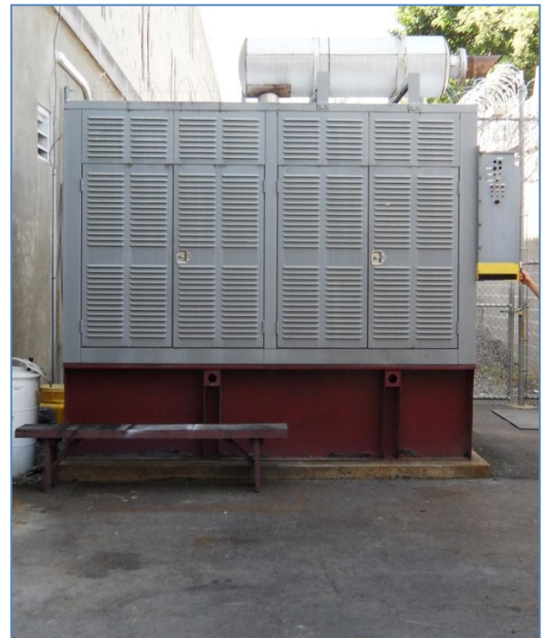
Existing 400 kW emergency generator
