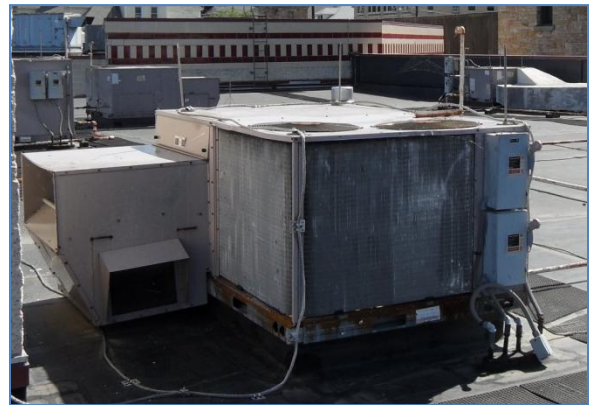
Typical Packaged Rooftop Unit
