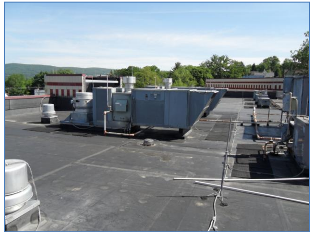
Existing hood make up air units
