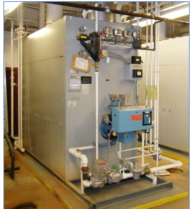
Existing Bryan Boiler
