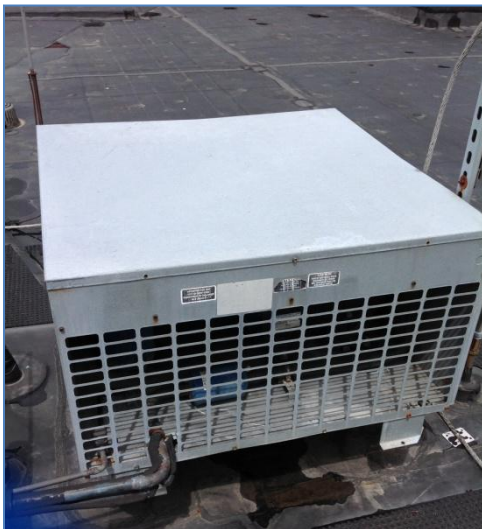
Existing condensing unit
