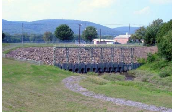
Wyoming Valley Levee System at Outlet of Abrahams Creek in West Wyoming Borough, Luzerne County
