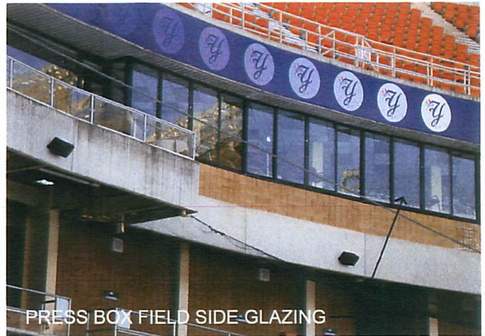
SPALLED / CRACKED CONCRETE AT LOWR BOWL WHEELCHAIR PLATFORM
