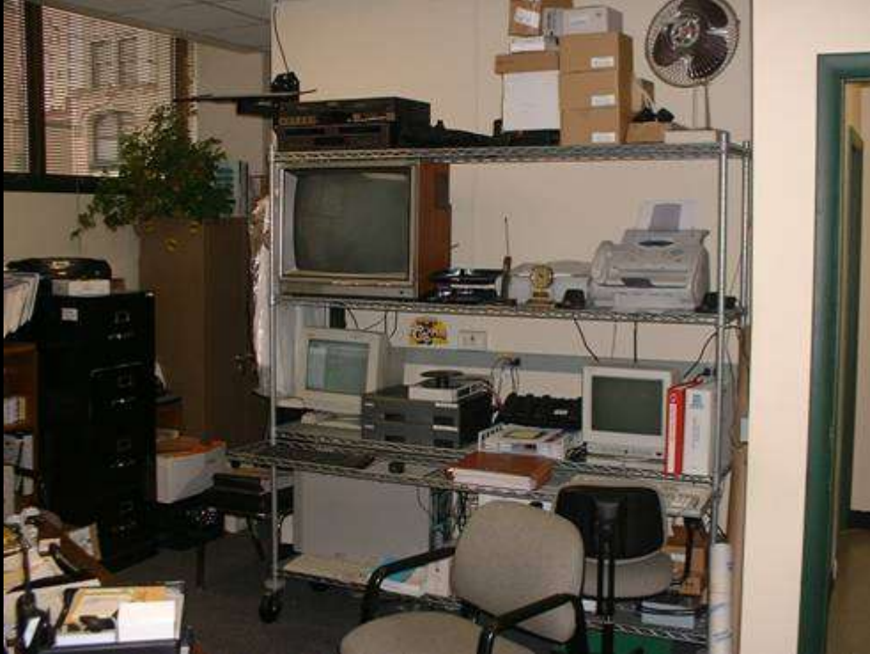
CPU Control Room
